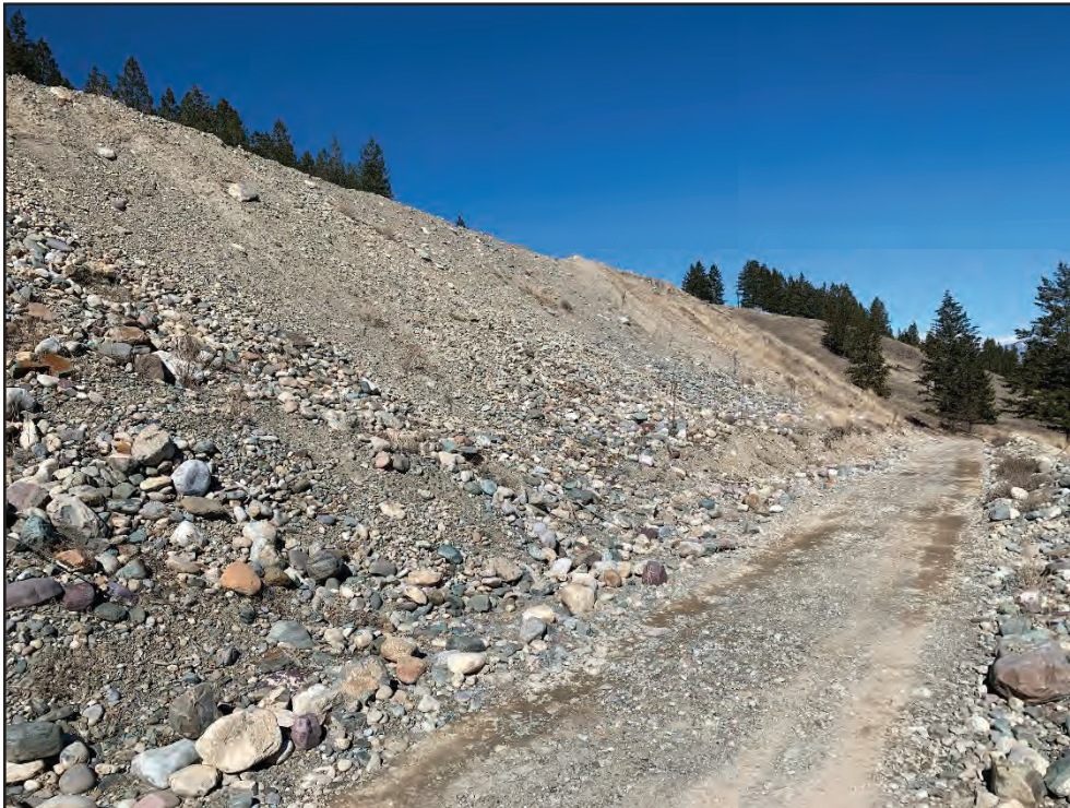
Photo 6: View of oversteepened granular fill slope, looking northerly. Material is very coarse. Slopes locally exceed 35 degrees (March 16, 2021).
