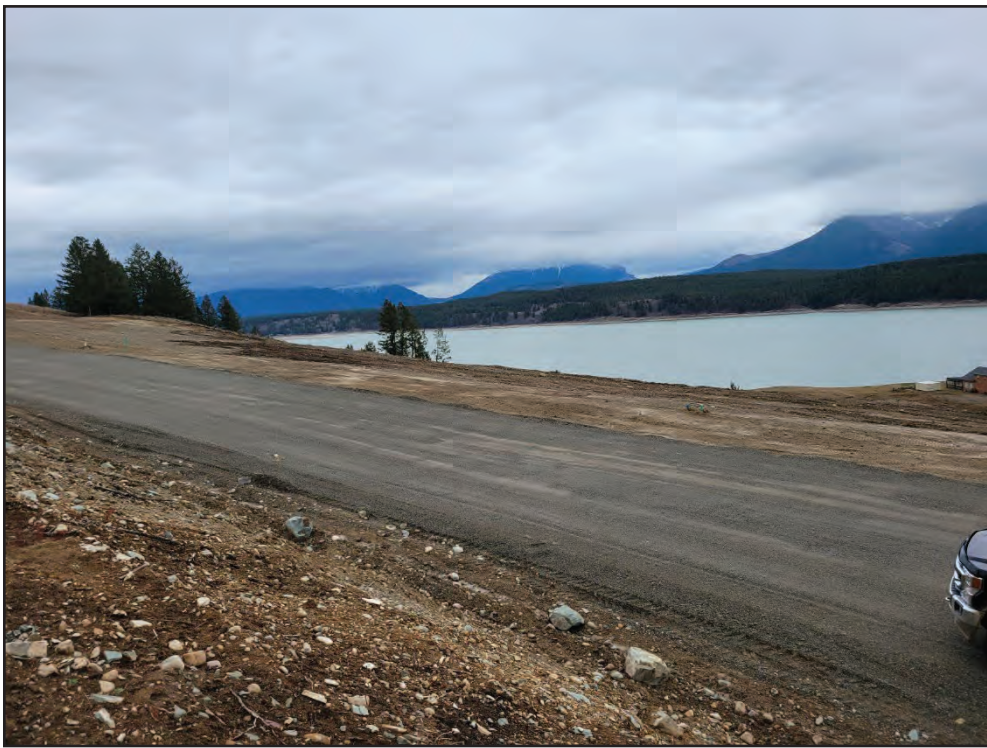
Photo 18: Central roadway between southern and northern areas following final rough grading. Photo by E. Mueller (November 30, 2021).
