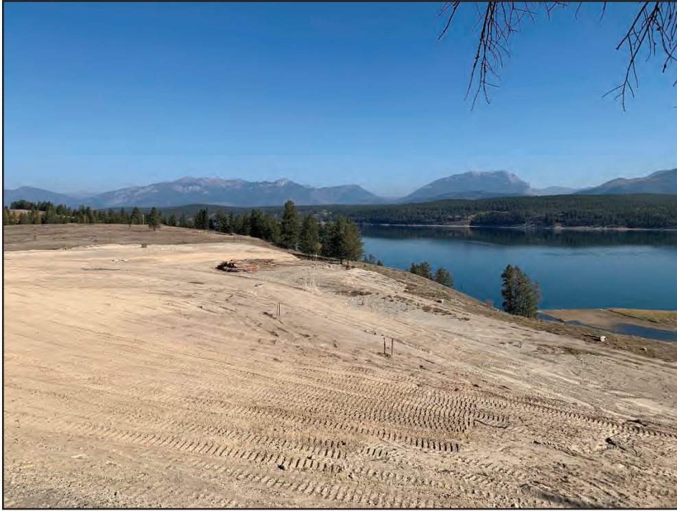
Photo 11: Middle Terrace Phase 2. Recently graded Lots 74 to 76 in northern area, looking to the northeast. Fence along north boundary of overall development can be seen in distance (October 19, 2021).
