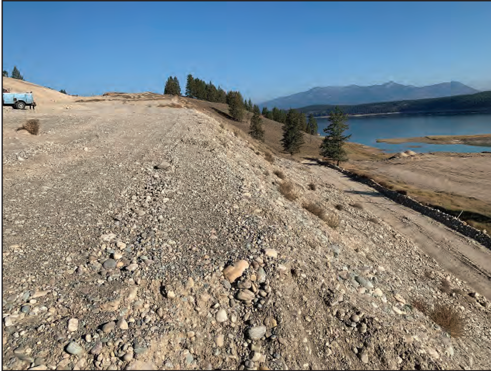
Photo 7: Middle Terrace Phase 2. Looking north along crest of east-facing slopes on Lots 72 and 73 in southern area (October 19, 2021).
