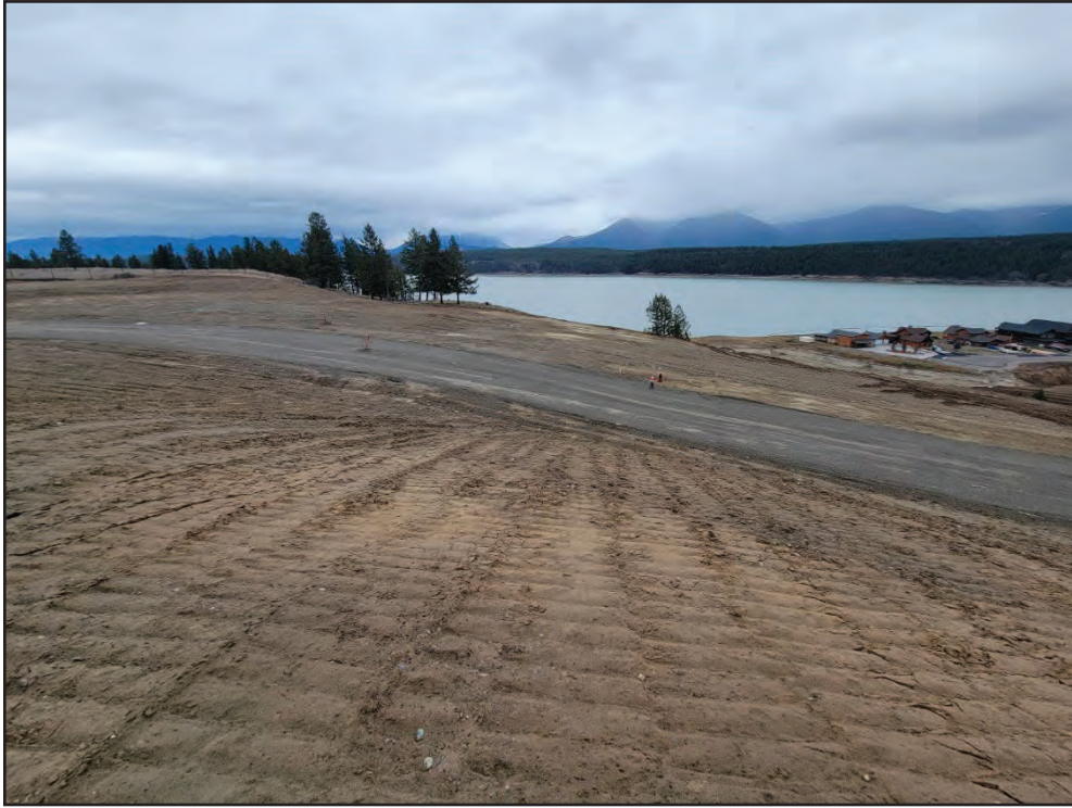
Photo 19: Middle Terrace Phase 2. Looking to the northeast across central roadway towards Lots 74 to 76 in northern area, following final rough grading. Photo by E. Mueller (November 30, 2021).
