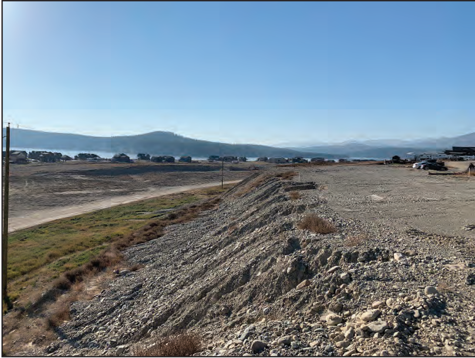
Photo 5: Middle Terrace Phase 2. Badly eroded/locally sloughing granular fill on east-facing slope in southern area (October 19, 2021).
