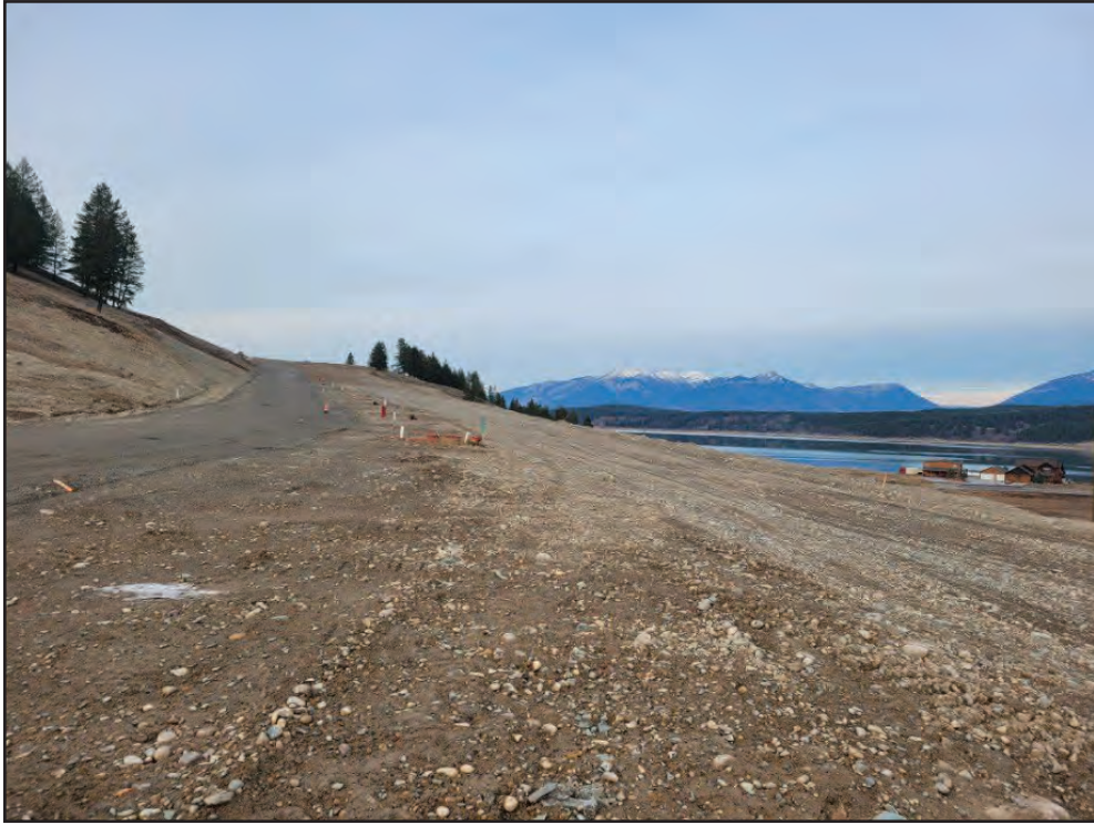
Photo 15: Middle Terrace Phase 2. View of graded lots in southern area, looking northward, with central roadway on left, following final rough grading. Photo by E. Mueller (November 30, 2021).
