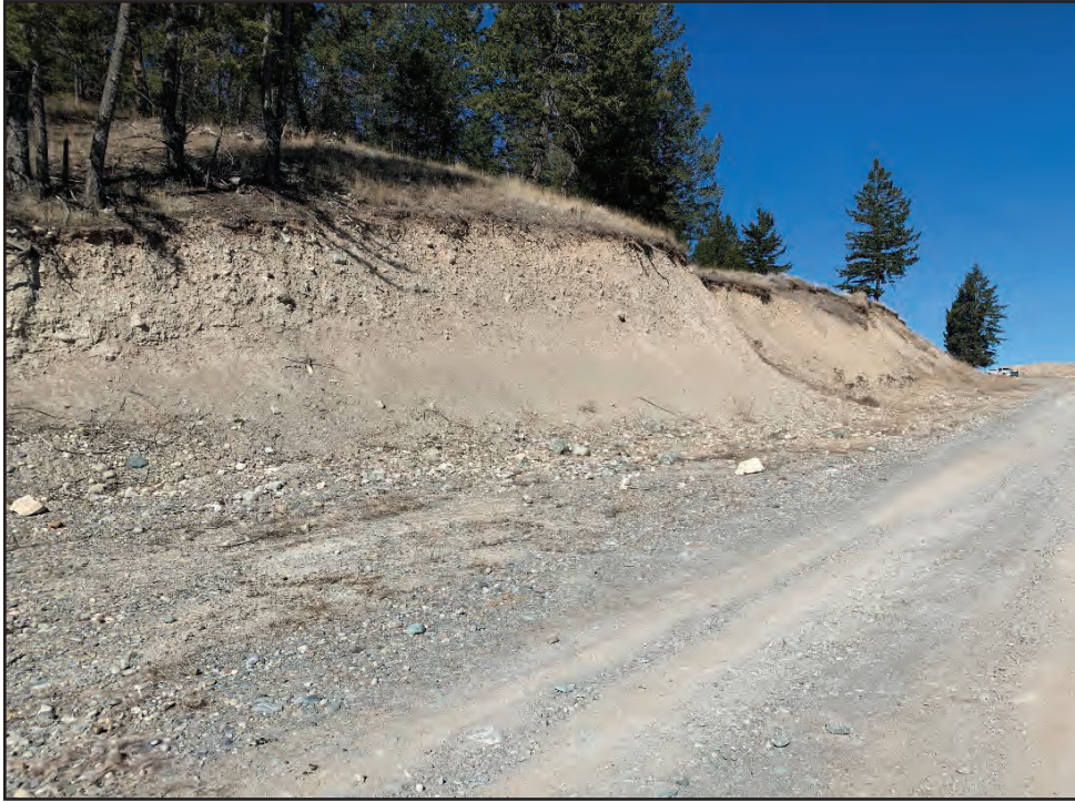
Photo 3: Middle Terrace Phase 2. Silty-sandy glacial till exposed in 3 to 4 m high road cut along west side of central roadway. Note talus (scree) accumulation along toe (March 16, 2021).
