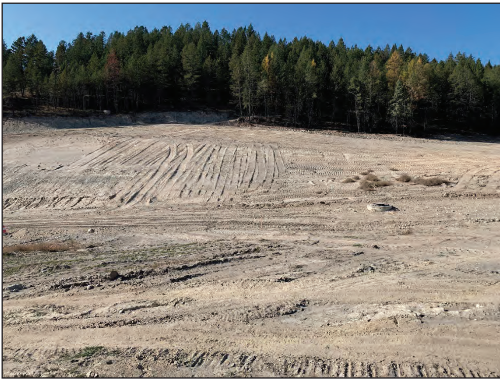
Photo 12: Looking west from central roadway at recently graded Lots 77 to 80 in northern area (October 19, 2021).
